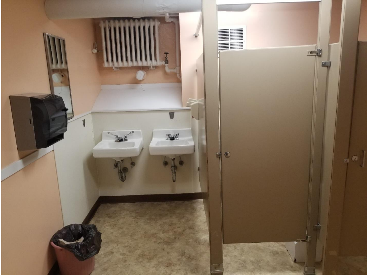
Restroom in basement level not ADA compliant
