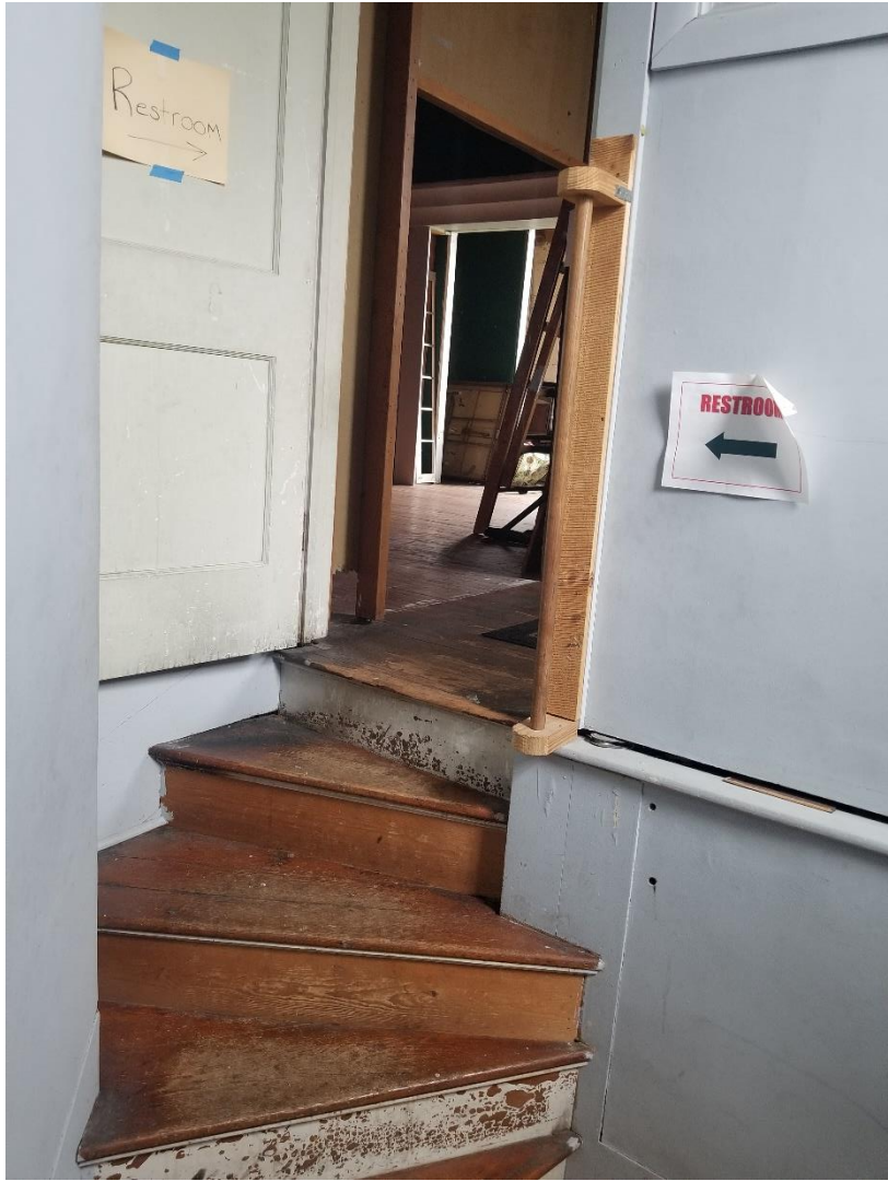
2 nd floor access to the restroom is not ADA compliant
